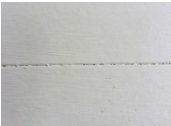
Post application inspection shows sheathing joint not properly sealed. Reseal with sealant.
